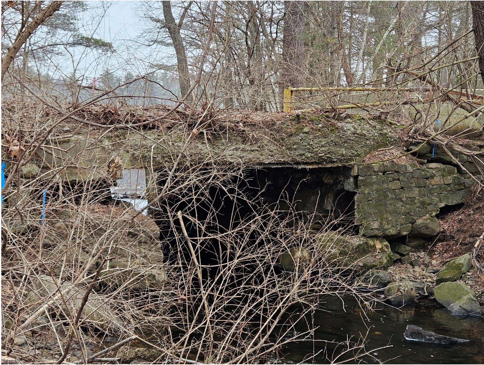
Photo 6: View of the Brandy Brow culvert from the downstream side facing north east.
