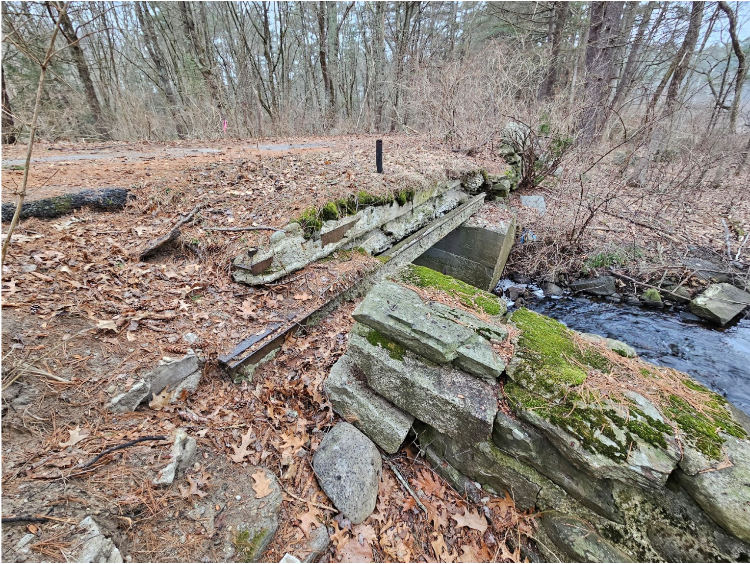
Photo 4: View of the top of the Brandy Brow culvert on the upstream side facing west.
