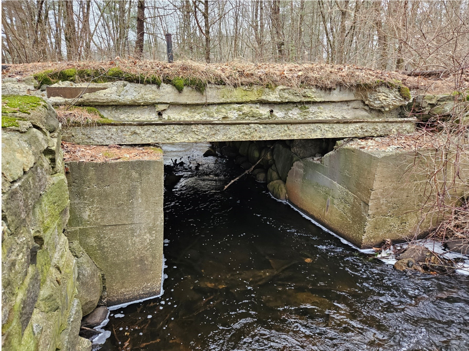
Photo 1: View of Brandy Brow Road over East Meadow River culvert on the upstream side, facing south.
