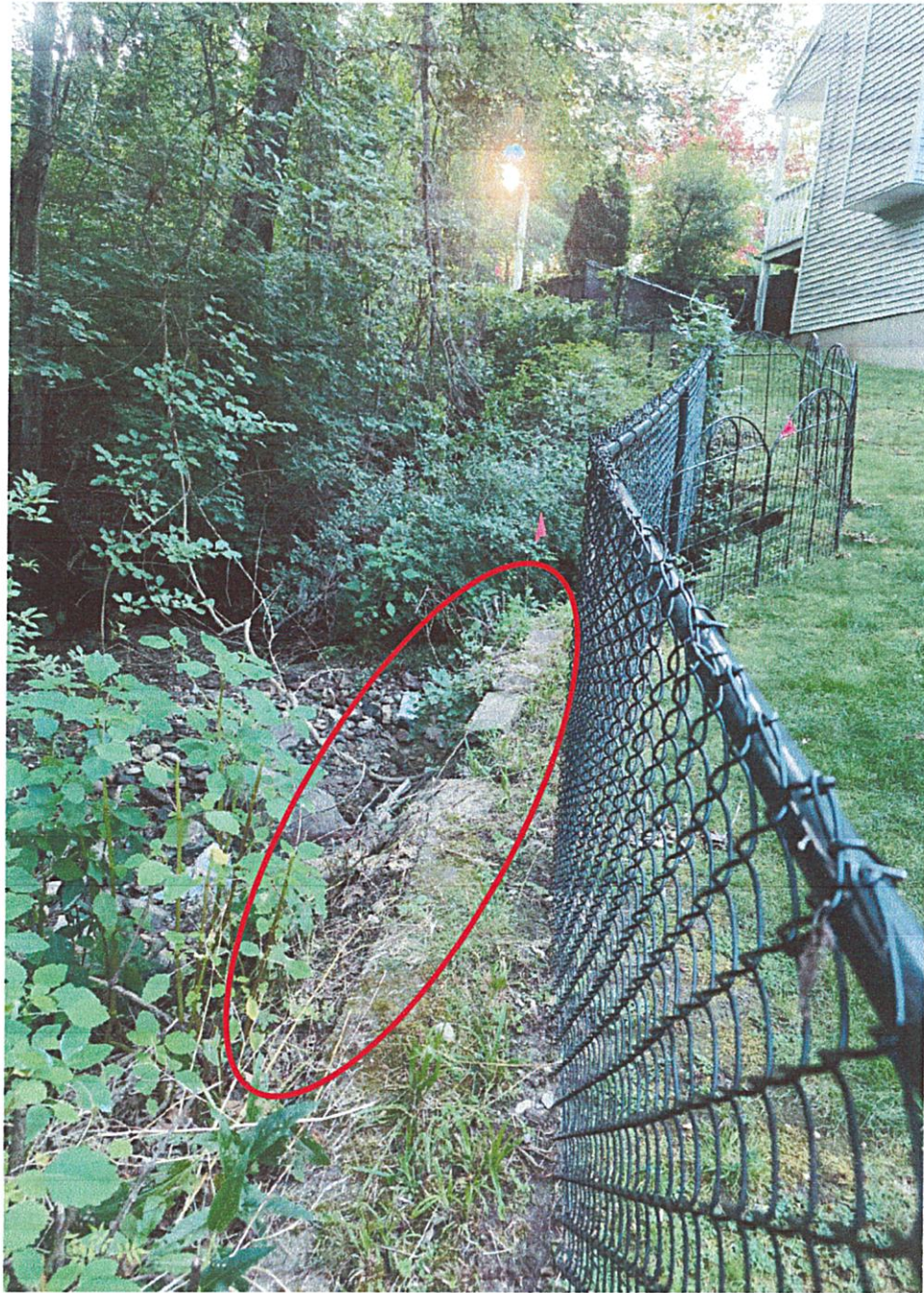
The original retaining wall is starting to fall and deteriorate.
